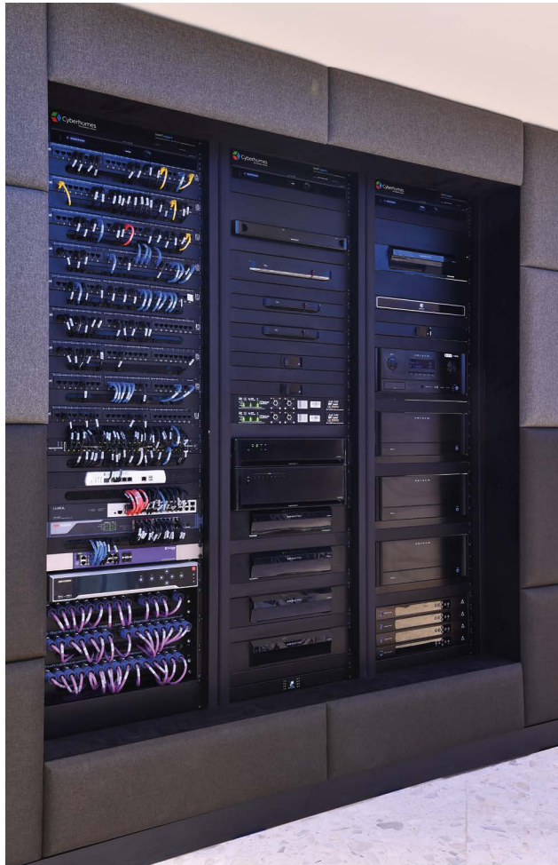
Dedicated AV racks in the basement plant room keep equipment out of the living spaces.
